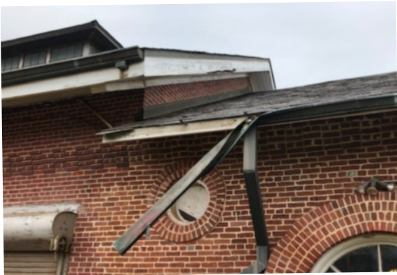
Gutter left hanging by the ice
