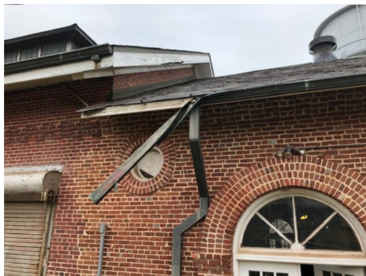
Twisted & hanging gutter knocked loose by ice.
