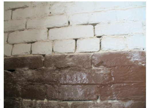
Closer look at a wall. Gaps between the bricks are not desirable!
