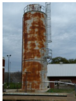
Lime tank "before"
