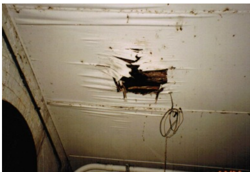
Ceiling in old office
