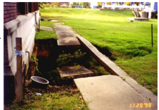
Sidewalk-eating sinkhole next to building
