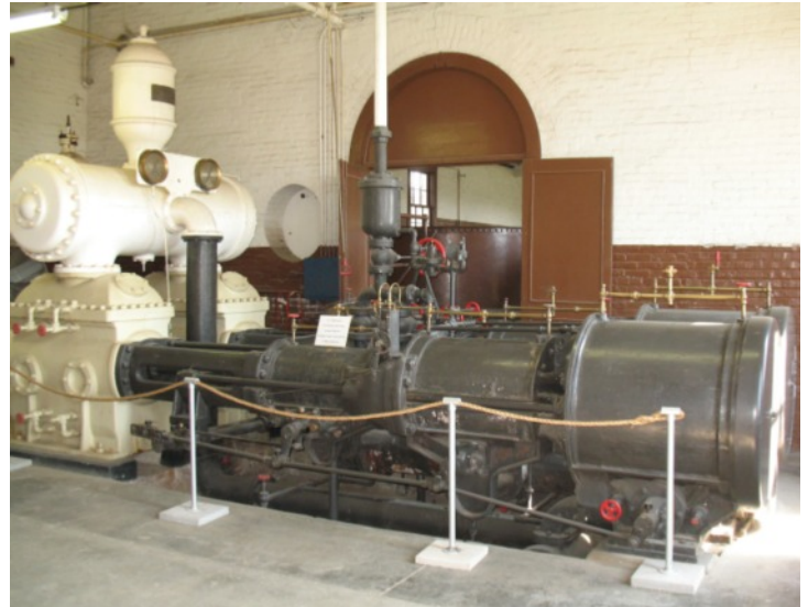
Worthington No.1 High Service Pump
