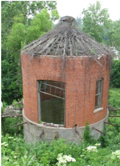
ca. 1911 Low Service Pumphouse Is there a steam pump in here?
