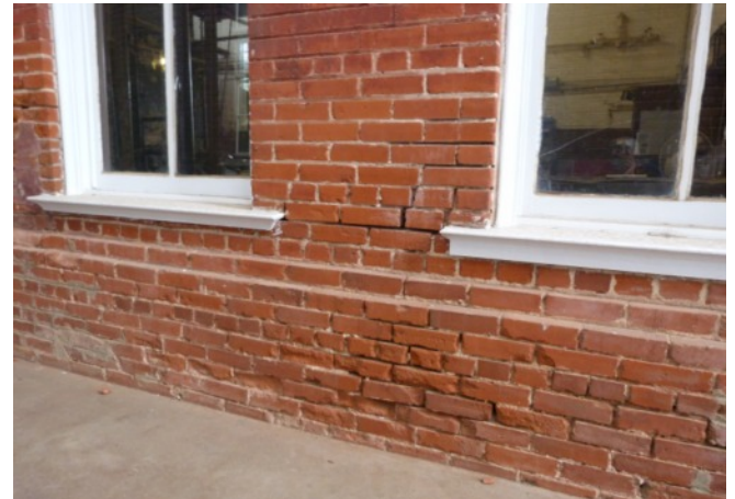
North Wall of Boiler Room Needs Repointing
