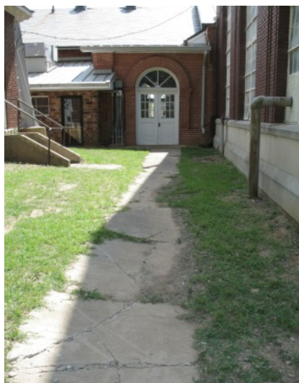
Sidewalk Needs Repair
